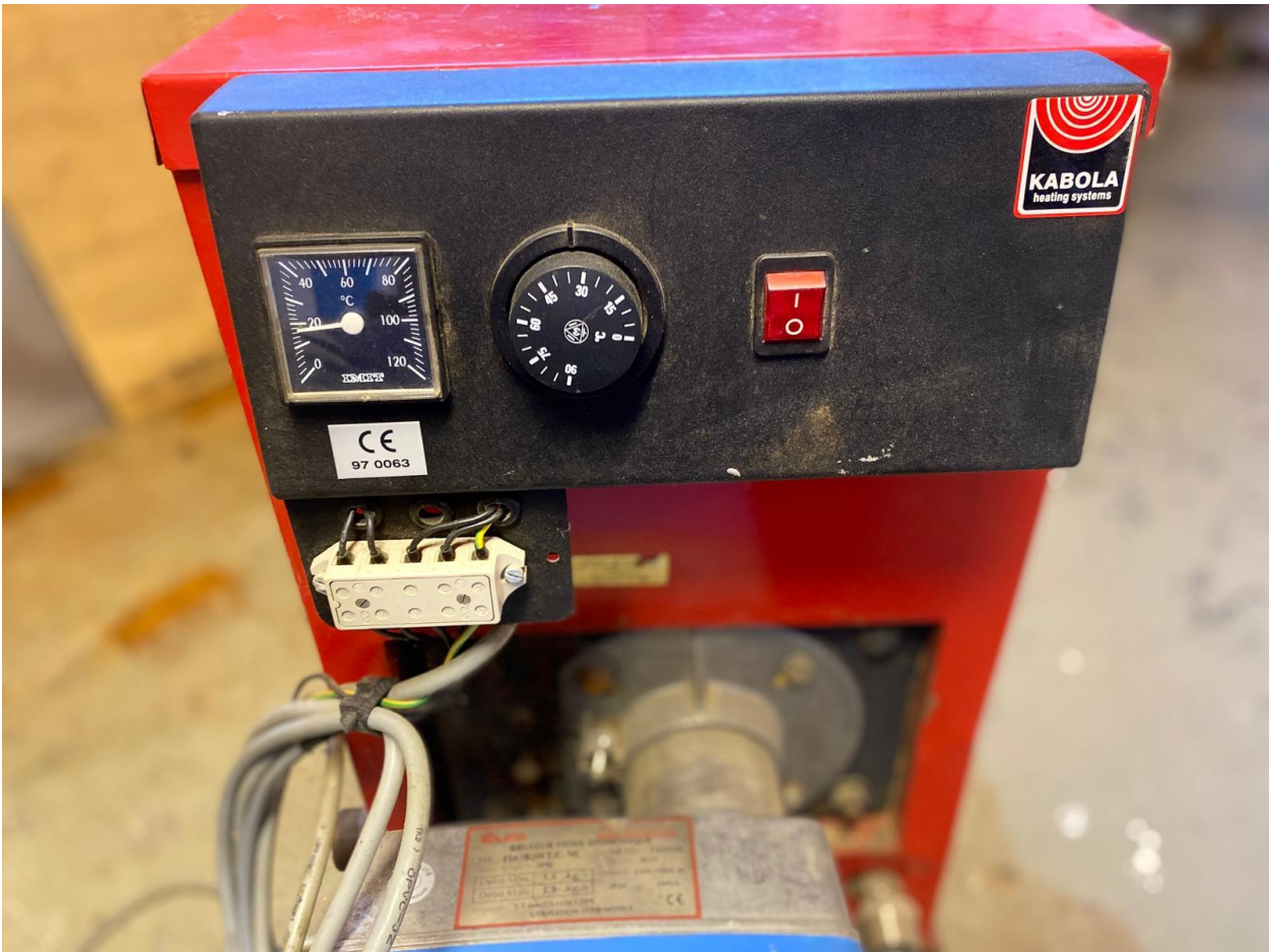
Figure 19 – Kabola Diesel Fired Boiler
