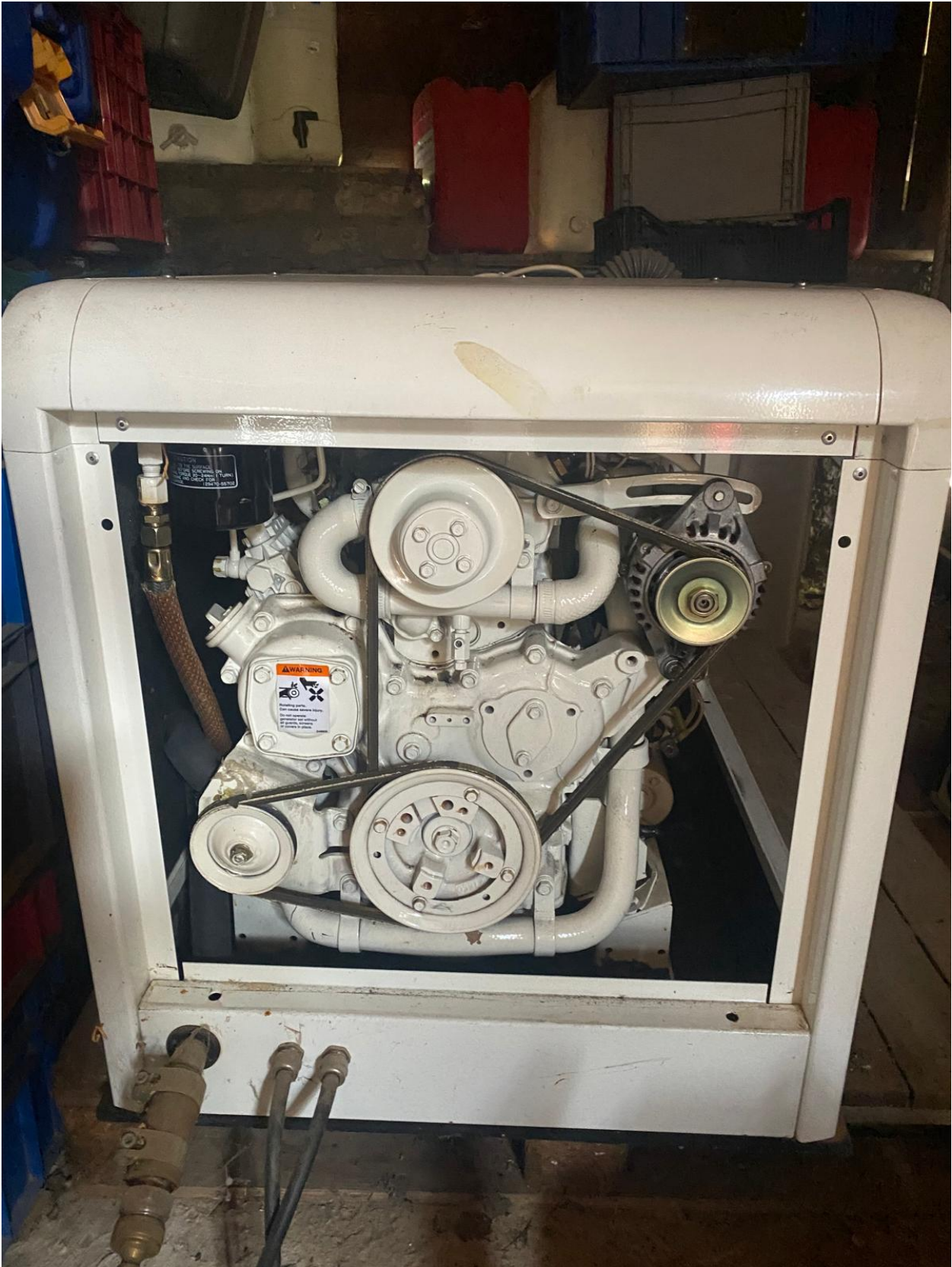
Figure 50 –Front of the Kohler Generator, cover removed.
