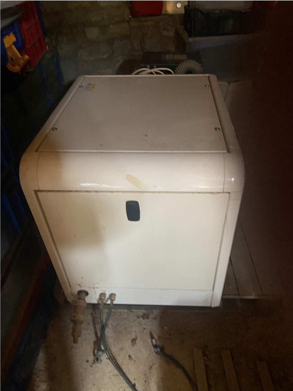
Figure 15 – Front of Kohler Generator, Cover in place.
