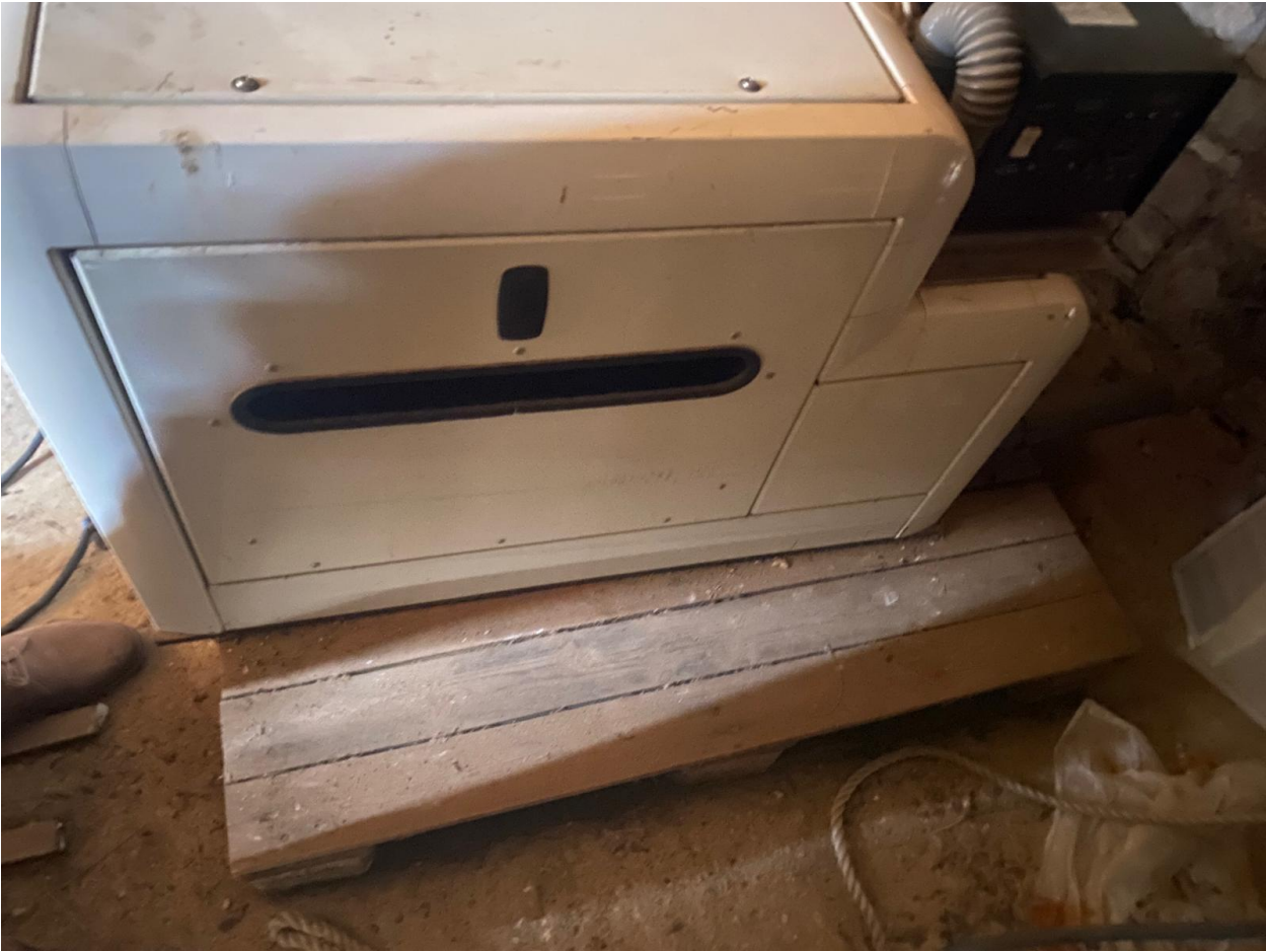
Figure 14 - Kohler Generator Cocoon, left side.
