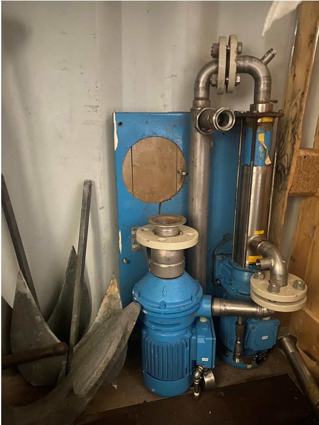
Figure 18 – Part of the Hamman Sewage Treatment Plant
