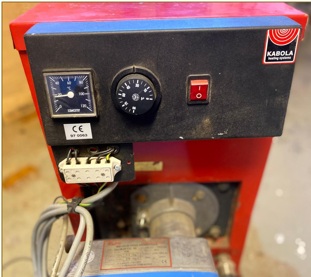
Figure 61 – Kabola Diesel Fired Boiler
