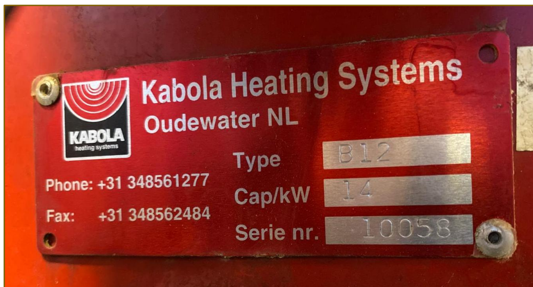
Figure 62 – Kabola Diesel Fired Boiler Nameplate
