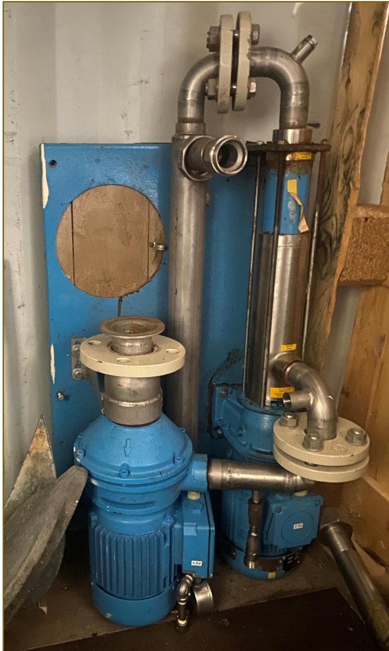
Figure 60 – Part of the Hamann Sewage Treatment Plant
