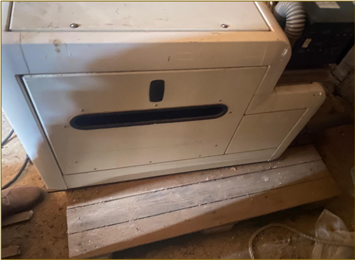
Figure 55 - Kohler Generator Cocoon, left side.
