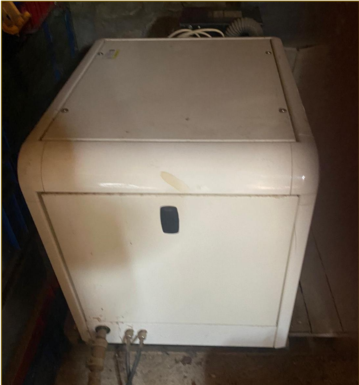
Figure 56 – Front of Kohler Generator, cover in place.
