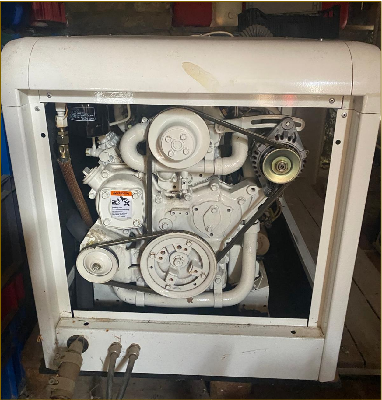
Figure 54 –Front of the Kohler Generator, cover removed.
